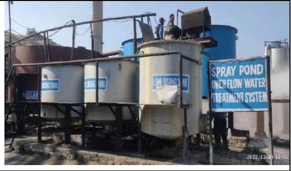
Pic.-16.Flow meter at main inlet channel of ETP
