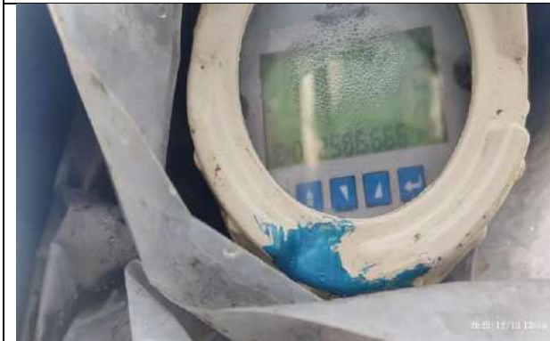
Pic.-19.Flow meter at centrifugal wash water
