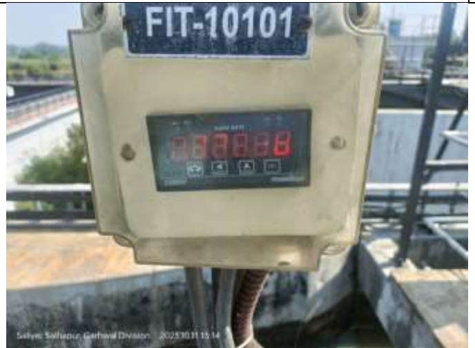
Fig 2: Inlet flow meter
