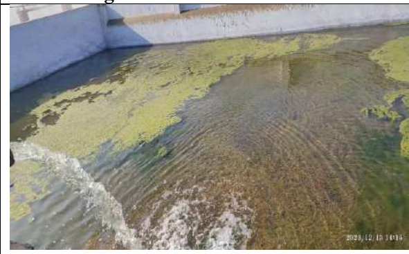
Pic.-14.Spray pond overflow treatment unit
