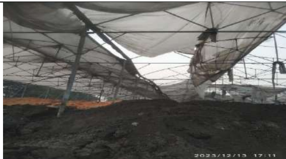
Photo 17: Damaged shed in bio-compost yard
