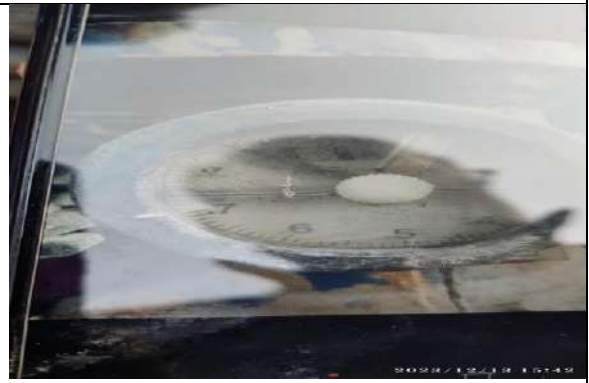
Pic.-20.Leakages in fresh water pipeline
