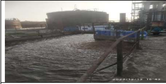
Photo 11: Aeration tank in CPU
