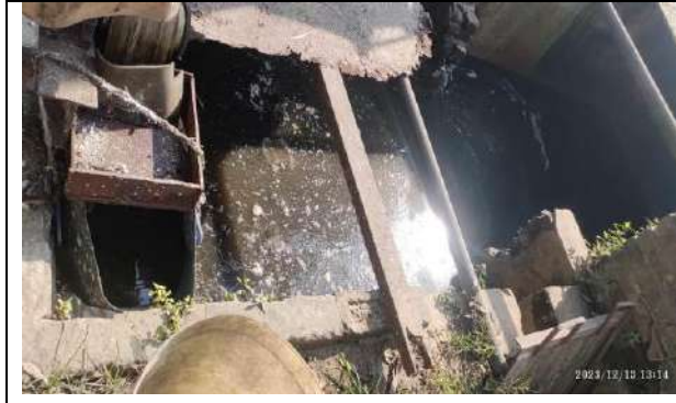
Pic.-07.Equalization tank without air mixing arrangement
