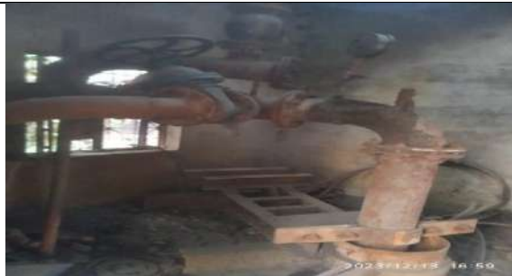
Photo 15: Borewell in distillery plant
