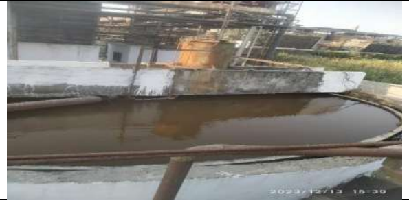
Photo 12: Secondary clarifier in CPU
