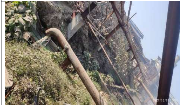
Pic.-17.Flow meter at inlet of SRS
