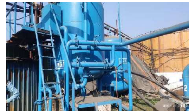
Pic.-13.Sludge drying bed
