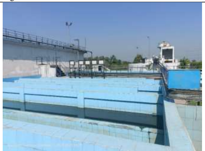
Fig 4: Chlorine contact tank
